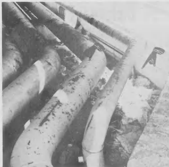
An assortment of rags, paper, cans, cartons, etc. along the full length of the pipe alley north of LCAR. Un surtido di panja biew, papel, bleki, caha, etc. den tur e largura di pipe alley pa noord di LCAR.
